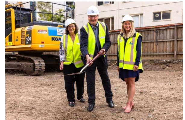
Mayor Heather Cunsolo (pictured right) joined Victorian Member for the Southern Metropolitan Region John Berger, officially representing Housing Minister Harriet Shing, and St Kilda Community Housing Chair Liz Johnstone for a ceremonial sod turn at the Wellington Street Site
