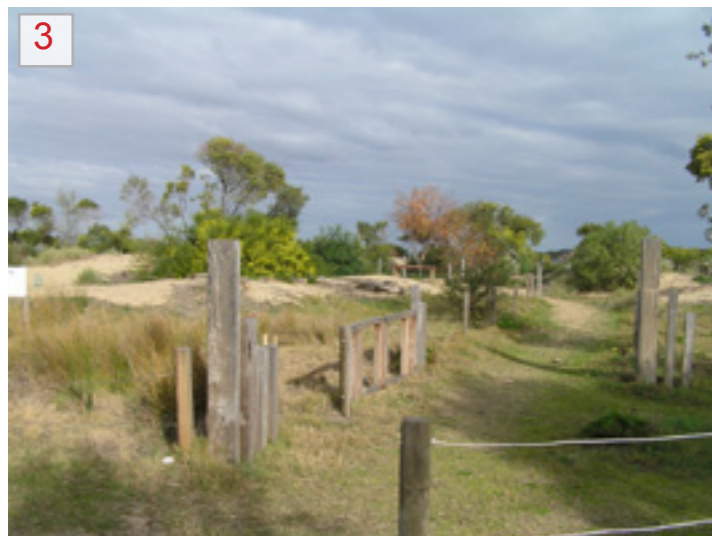
3 Current reserve entrance (west of LSV building) - Typical fence and path. Through the middle of the photo there are areas lacking vegetation cover. Fences require repair and paths require upgrading/renewal.
