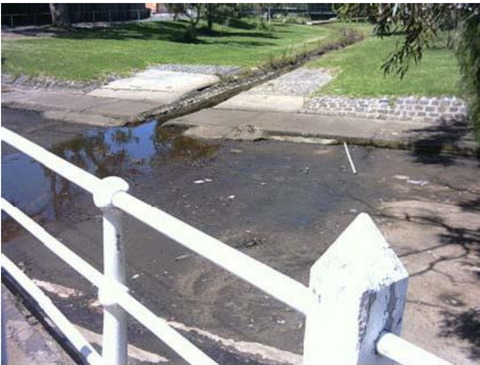
Figure 6.26-4 – Looking south from Glenhuntly Rd bridge, showing start of the Elsternwick Main Drain
