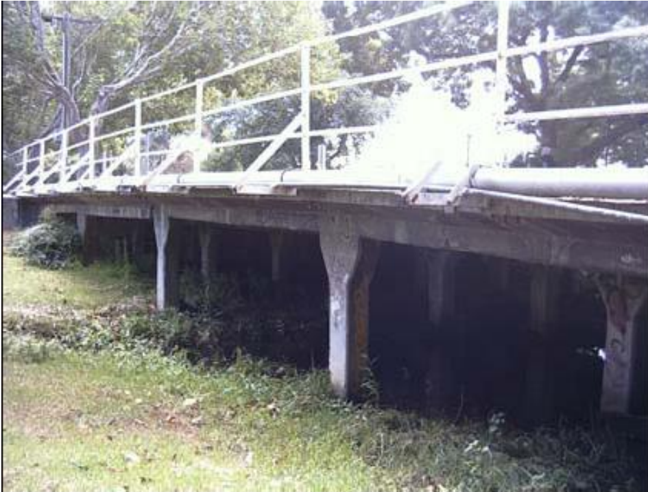
Figure 6.26–5 – Reinforced concrete girder bridge at St Kilda Street, designed by John Monash
