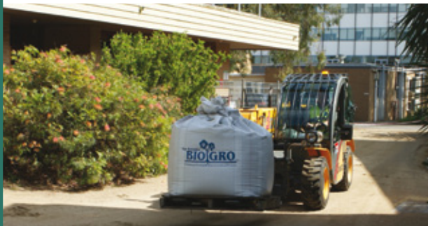
Bulker bags of substrate moved around the site, at ground level, prior to being lifted by crane at the demonstration roof at The University of Melbourne's Burnley campus
