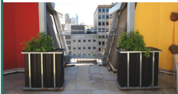
Planter boxes on the City of Melbourne's Council House 2 roof garden, Little Collins Street, Melbourne, have not performed as well as expected
