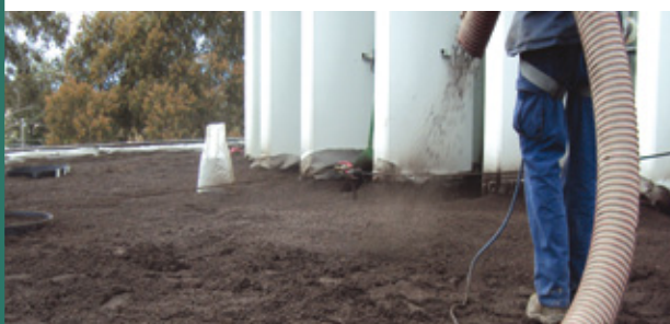
Substrate was blown onto the green roof in the City of Monash, Glen Waverley. Image Junglefy
