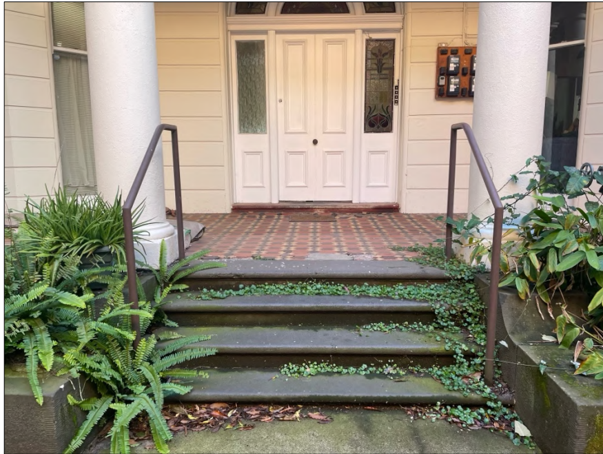
Figure 7 Front steps to the former mansion. The steps may be early or original fabric, with non-original handrails.
