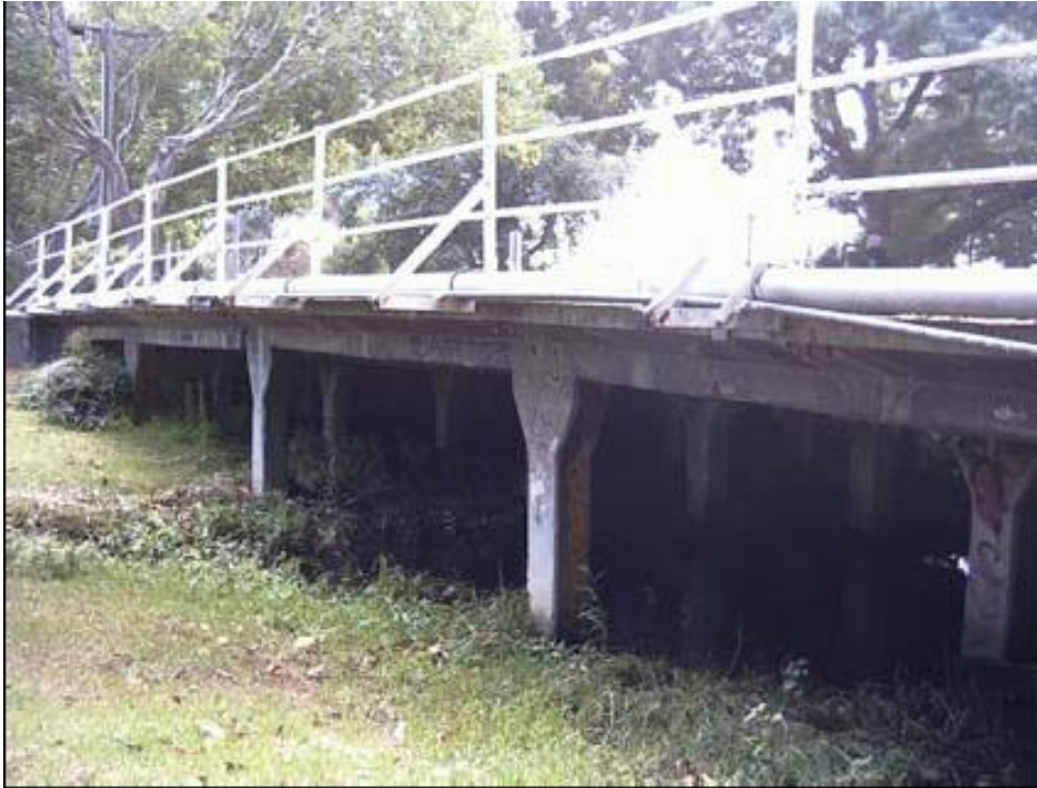
Figure 6.26–5 – Reinforced concrete girder bridge at St Kilda Street, designed by John Monash
