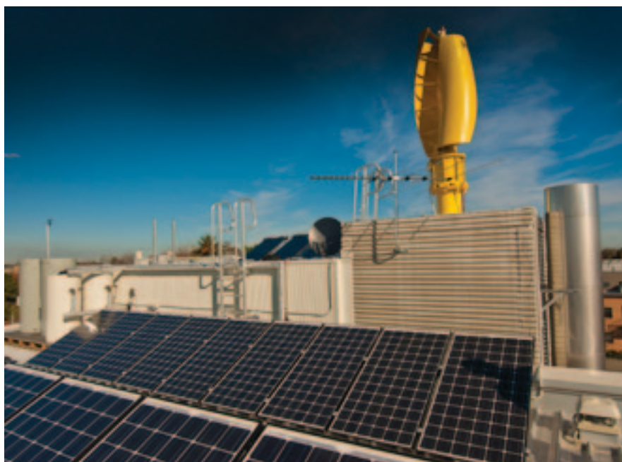
Renewable energy technology is a growing source of energy for our larger residential and commercial buildings, such as this recent apartment block in Elwood.
