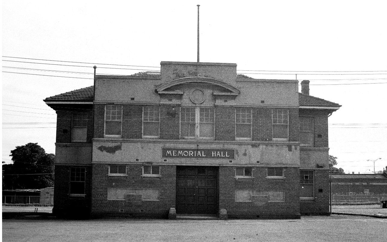
Figure 18, Front façade of the Memorial Hall, c1970-74. Note the peeling paint and render. (State Library of Victoria, Committee for Urban Action Collection)
