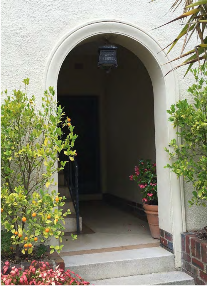
San Bernards - detail of the porch showing original wrought iron light fitting with San Bernards etched into the glass, terrazzo floor and wrought iron balustrade to the staircase.
