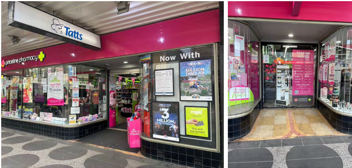
Original shopfronts to Acland, showing (at right) terrazzo floor to the ingos (covered by mat in left image)
