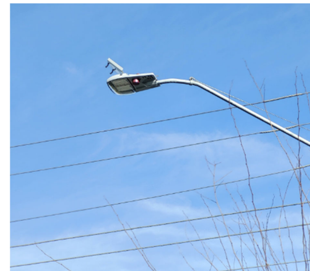
New LED street lighting
