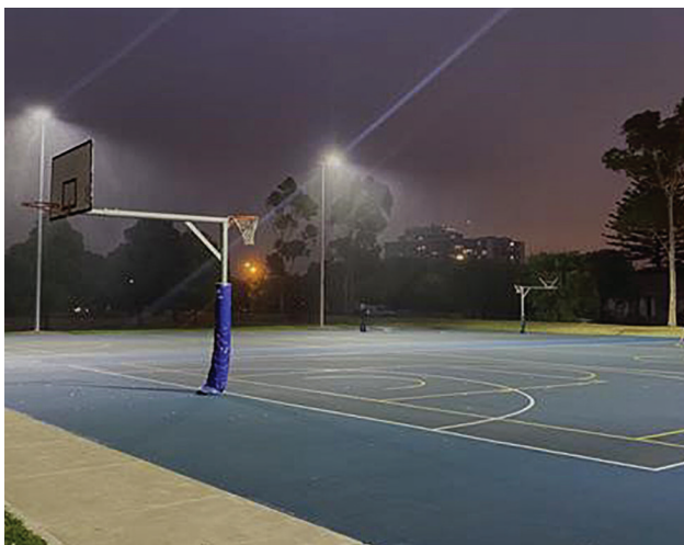
RF Julier Reserve netball court lighting
