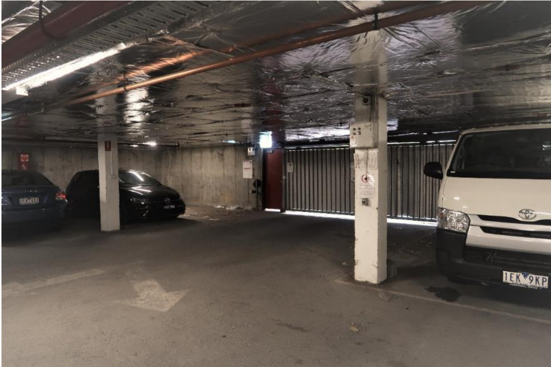
Figure 20 Basement parking area (LG.02) with sliding gates to Duke Street evident at rear
