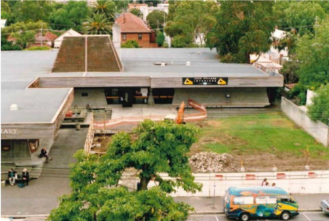
Figure 12 St Kilda Library south elevation, part, c. 1994 during construction of the additions Source: City of Port Phillip History Collection
