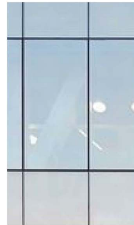
GLA02 Silver Pewter Glazing Total glass/frame system to achieve thermal performance as required by ESD and Facade consultants Max reflectivity 20%
