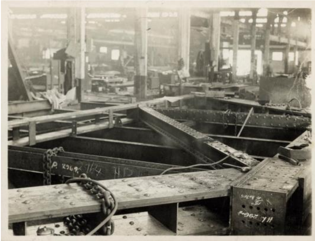
Figure 36: Large riveted and welded truss in course of fabrication in Johns & Waygood's shop, 1935, Stephenson & Meldrum Architects. H92.374/71, Sennitt's Premises Sth. Melb.
