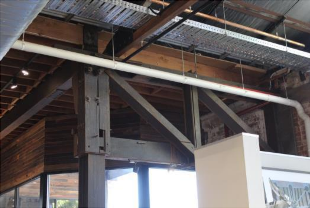
Figure 24: Braced support to front
