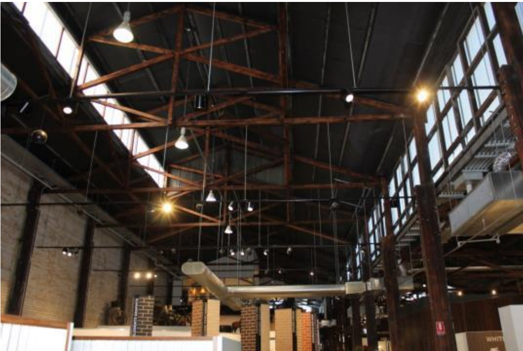
Figure 25: Interior timber work showing roof trusses, posts and later brick party wall on west side
