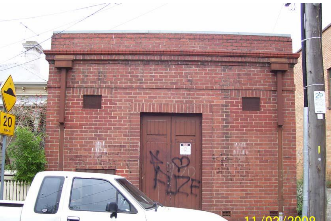
Figure 51: MCC substation Nottingham Street, south of Racecourse Road, Flemington.
