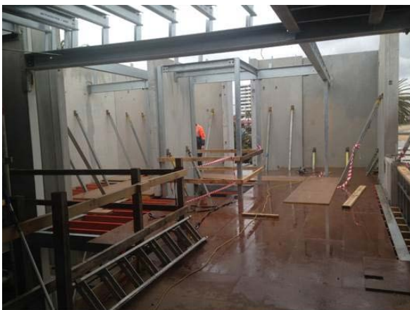
Concrete panels and structural steel now installed at St Kilda Life Saving Club
