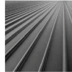
F17 ROOF SHEETING Lysaght Klip-Lok 700 Hi-Strength to pavilion roof. Unpainted Zincalume Finish.
