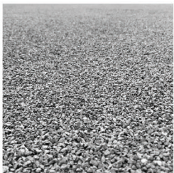
F18 BALLAST ROOF Ballast roof finish to the roof of the southern pavilion.
